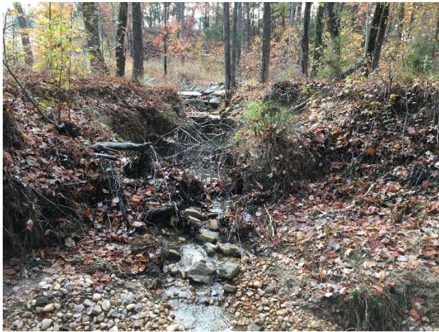
Headcut looking upstream
