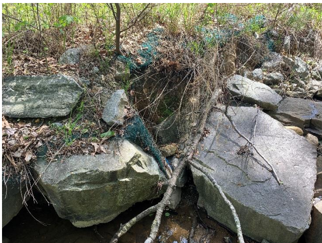
Void behind structure rock due to high flows along S12.
