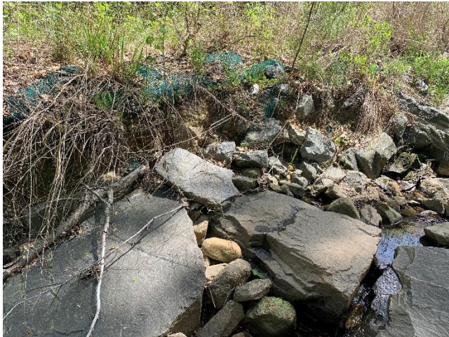
Bank erosion from high flows flanking S12.
