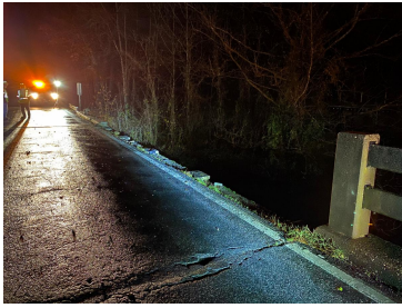
Photo 1: Damage during the vehicle crash collapsed and pushed the bridge's outer retaining barriers on the northbound side off the bridge.
