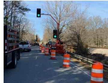
Photo 3: Crews installing temporary automated control systems that will guide one-way traffic across the bridge.
