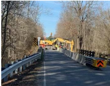
Photo 2: Bridge crews work to install temporary retaining walls to allow for one-way traffic while repairs are completed.
